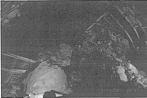
Figure 1. Collapse of tunnel roof in Qazvin-Rasht seventh tunnel.
