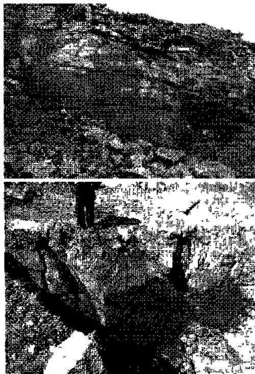
Figure 2. Blast damage to the bench walls, (a) increased fracturing near crest of bench and (b) loosening of rock wedges and loss of bench width.
