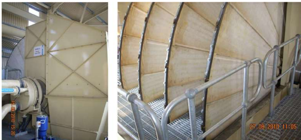
Figure 3. Disc filter (176 m 2 filter area) assembled in the gold/copper mine; view of control head side (left); and view of the four filter discs with walkways (right)
