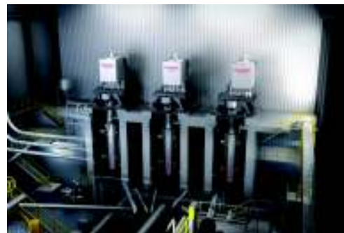
Figure 3. Typical HIGmill Installation - 3 x 5MW
