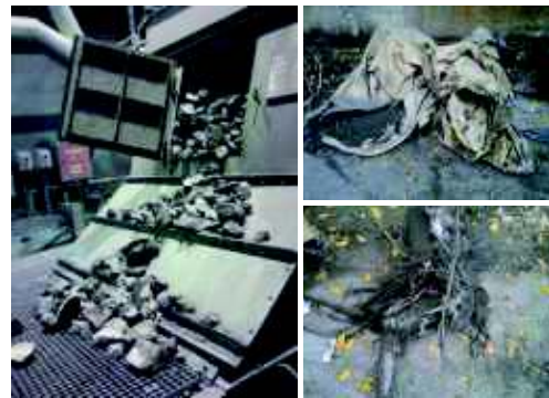
Figure 13. Photos showing cone crusher and double deck screen plugs
